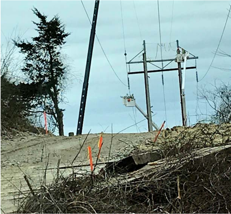
Three Phase Line Construction crews transfer an energized conductor from a wooden H-frame to a new, adjacent steel structure using the bare-hand method.
