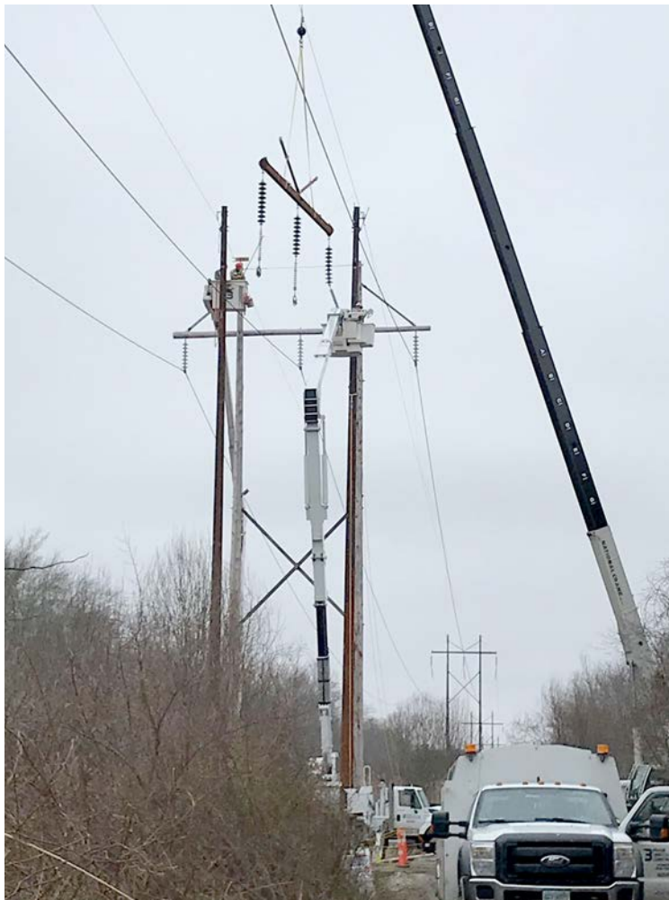
Using the barehand method, Three Phase Line Construction crews have set two new steel poles. They are also working to install a steel cross arm for one of the new H-frame structures on Eversource’s 1465 Line in Connecticut.
