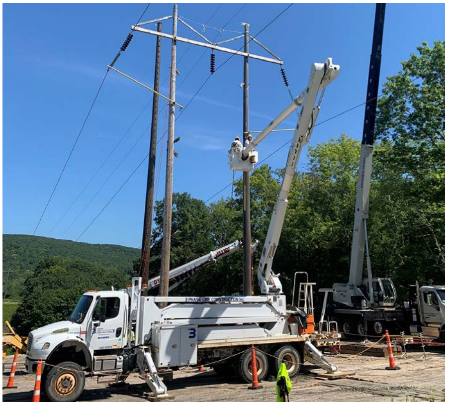
Three Phase Line Construction line workers undertake make-ready work on a conductor as part of setting a new H-frame structure.
